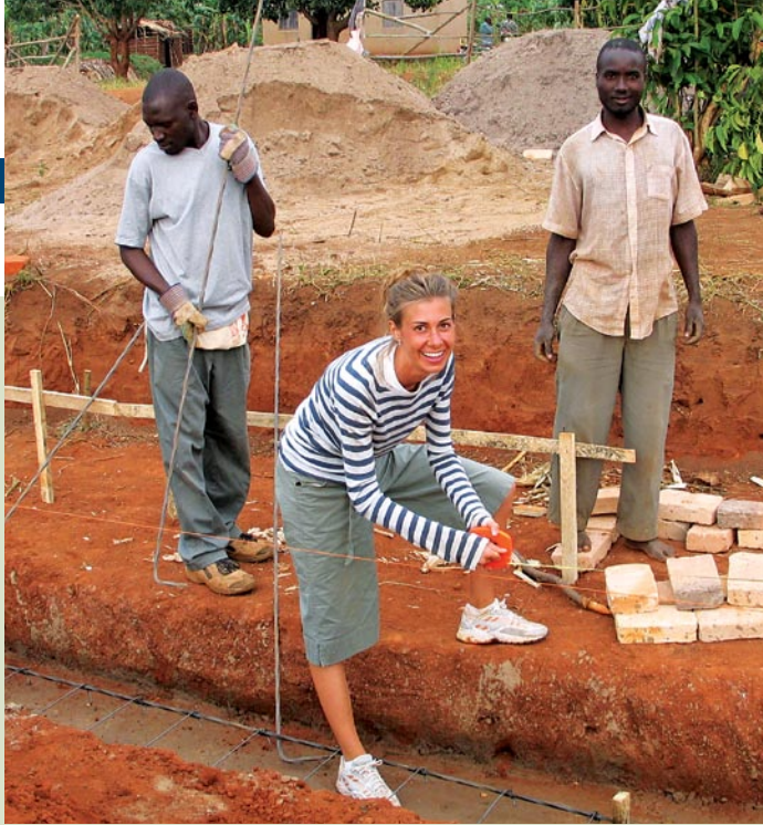
Stephanie Van Dyke '99 works with villagers in Ddegeya, Uganda, last summer as they prepare the foundation for a new clinic.
